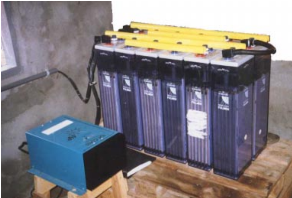
Photo 13: Deep cycle 'Solar' battery in Sri Lanka. Twelve 2 volt cells with 900 Ah capacity are connected to make one 24 volt battery with 900 Ah capacity. Height is 700mm. On the left is an inverter. (Hugh Piggott)
